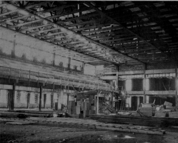
Exactly six months have passed since the "skeleton" of the gymnasium appeared in the Cowl, and this is what the gym looked like a few short days ago. Construction is moving at top speed with completion deadline this spring. —Cowl Photos by Fleck
