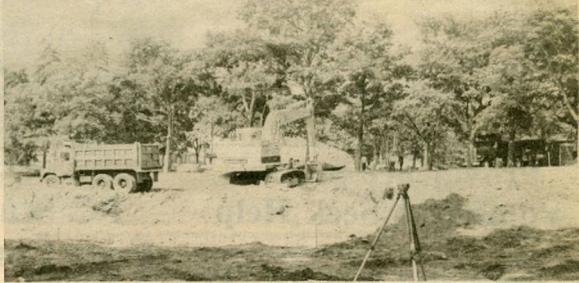
Construction of two new residence facilities on the corner of Huxley and Eaton street is currently underway to alleviate the housing problem on campus. (Photo by Joseph E. Gaines)
