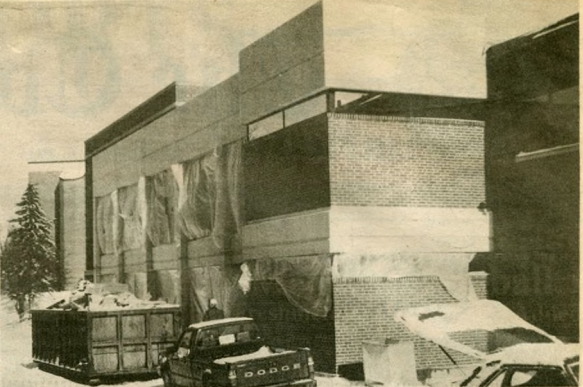
Construction of the connector building for the science department is finally ready for use after months of delays. (Cowl photo by Joe Gaines)
