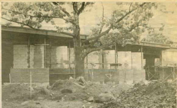
The new building for the Western Civilization program is currently under construction.
