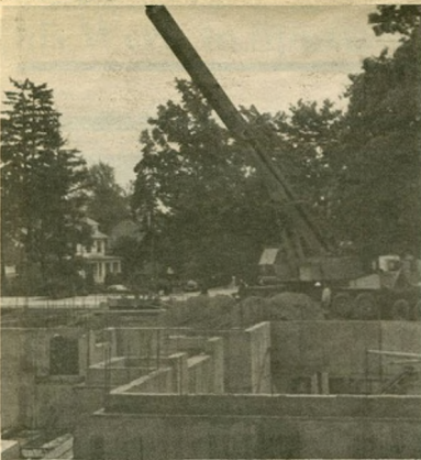
Progress continues on the construction of the new residence facilities. Shown here is the foundation work which is approaching completion. Photo by Joe Orroleva.
