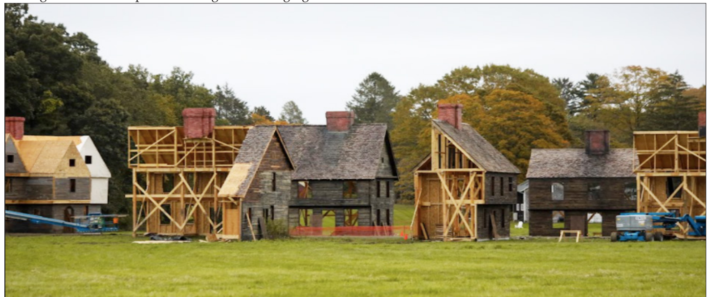
A set in Lincoln, RI being constructed for the filming of Hocus Pocus 2 .
